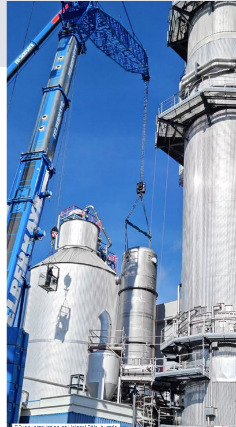
DEvap installation at Heinzl Pöls, Austria
